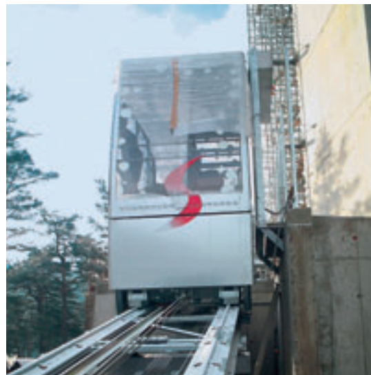
Application: Inclined lift to the ski jump at the Isel mountain, close to Innsbruck, with Loher DYNAVERT drive (inverter and motor) and SIMATIC S7 control
